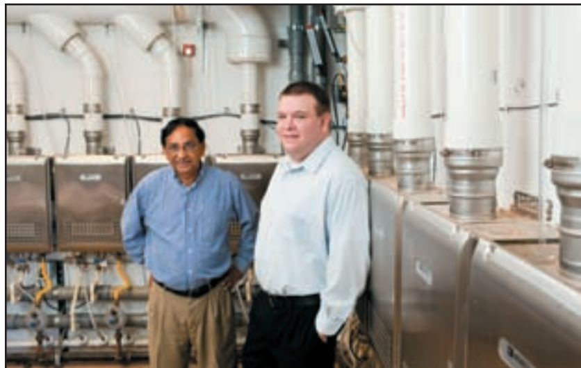
In the mechanical room are Giri Yadla (left), director of new construction & facilities management at The Residence Inn by Marriott; and Timothy Pritchett, general manager of the Florence, Ala., Residence Inn.
