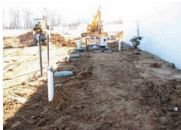
Commercial greywater systems can pull from sinks, condensation lines from HVAC systems and rooftops. This water is filtered and chlorinated and stored in tanks. Pictured above is a completed installation at a prison facility.
